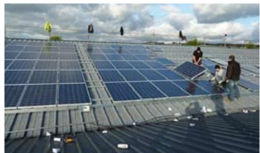
Solar panels (photo Greenerthenergy)
